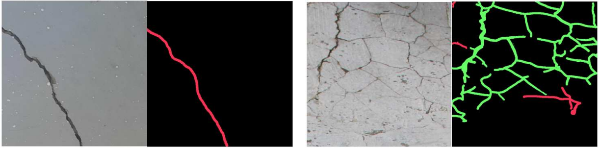
Fig. 4. Segmentation annotation: left — class crack, right — class web_crack
